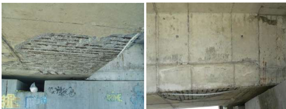
Figure 5. Affected areas of the bottom of the concrete girder.
